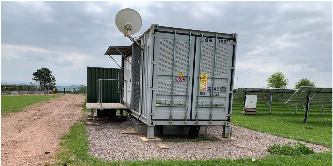
Photograph 14.19: Typical Inverter Container
