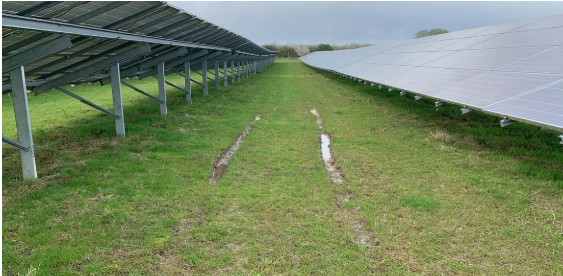
Photograph 14.24: Example of Minor Ruts Caused by Vehicles
