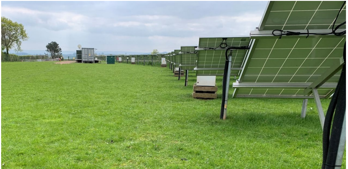
Photograph 14.18: Example of Buried Cables, Monmouthshire
