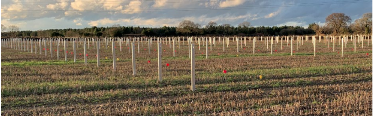
Photograph 14.12: Recently Installed Mounting structures (Tiln Farm, Retford, January 2023)
